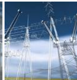
High-voltage switch gear
