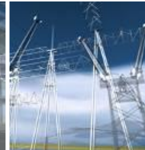
High-voltage switch gear
