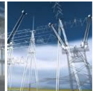
High-voltage switch gear
