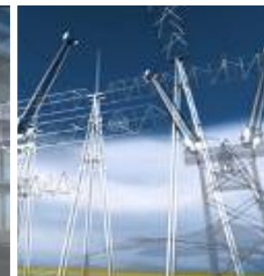
High-voltage switch gear
