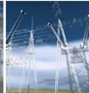
High-voltage switch gear
