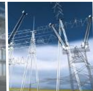
High-voltage switch gear
