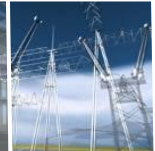
High-voltage switch gear
