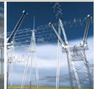
High-voltage switch gear
