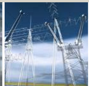
High-voltage switch gear
