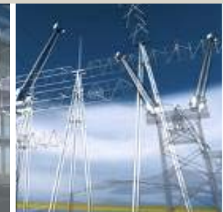
High-voltage switch gear
