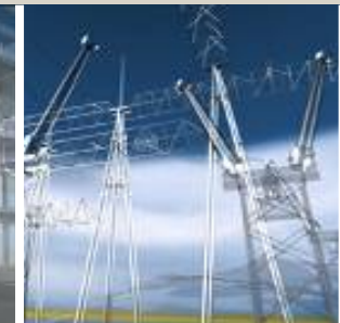
High voltage switch gear
