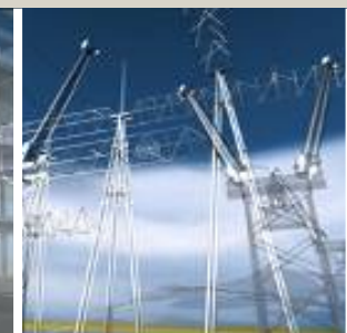
High-voltage switch gear
