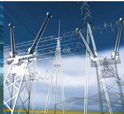
High-voltage switch gear
